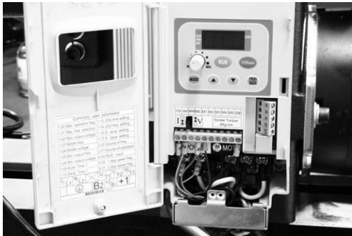
VFD with cover open
